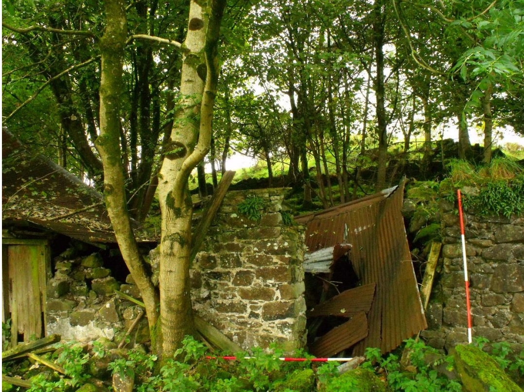
Plate 5: Photo of cottage showing poor state of preservation, looking west
