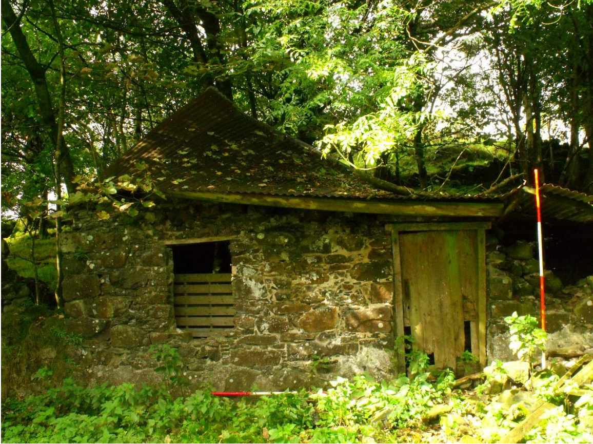
Plate 7: Façade of the building showing door and windows on either side, looking west
