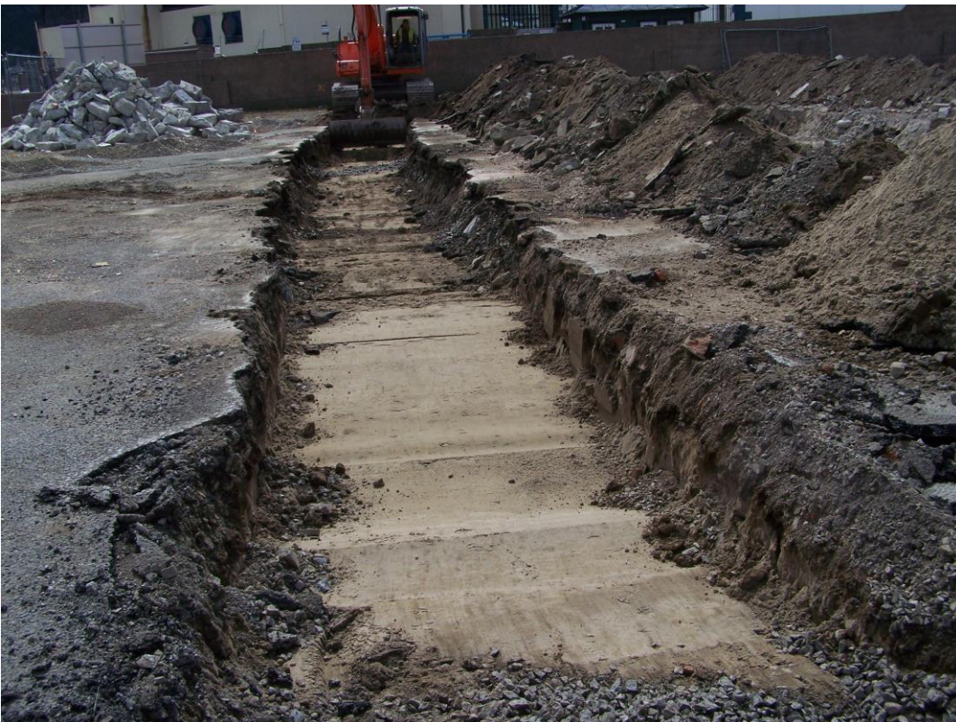
Plate 6: Trench 5 post-excitation (looking south-west). Note pile of stone near corner of site.
