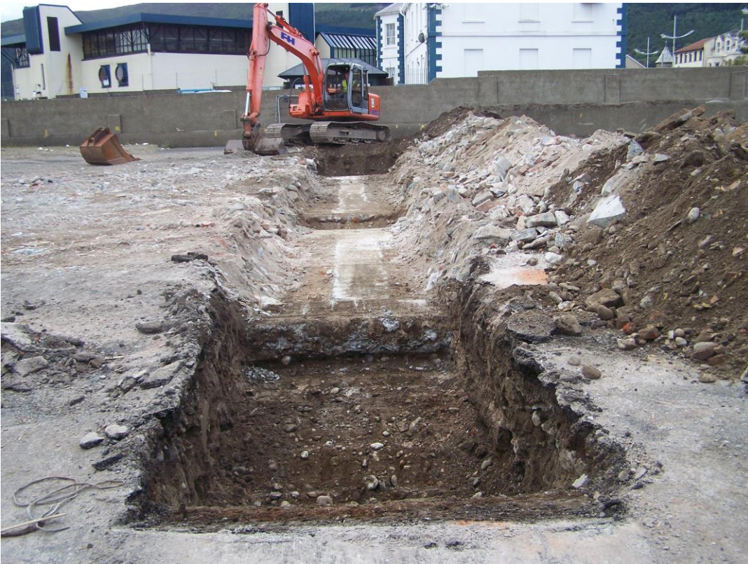
Plate 4: Trench 3 post-excitation (looking south-west). Note the concrete foundation footings running through middle of trench.
