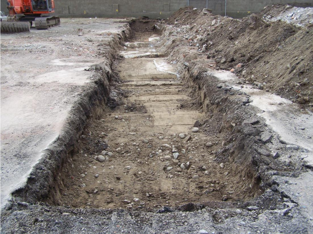
Plate 5: Trench 4 post-excitation (looking south-west). Note the concrete bay windows and porch footings.
