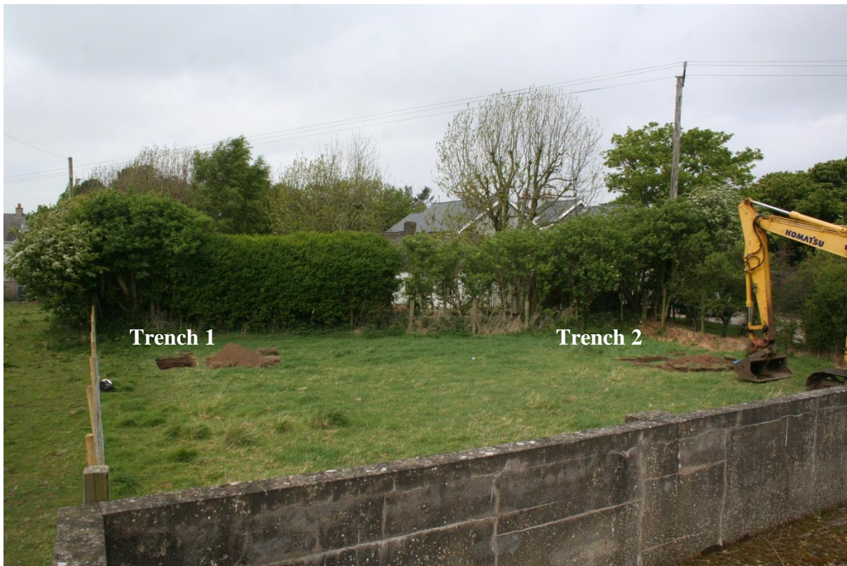
Plate 1 Photo of the application site (facing northwest) showing the location of the hand-dug trenches, Trenches 1 and 2, before they were extended mechanically. The western wall of the concrete cattle pen is visible in the foreground.
