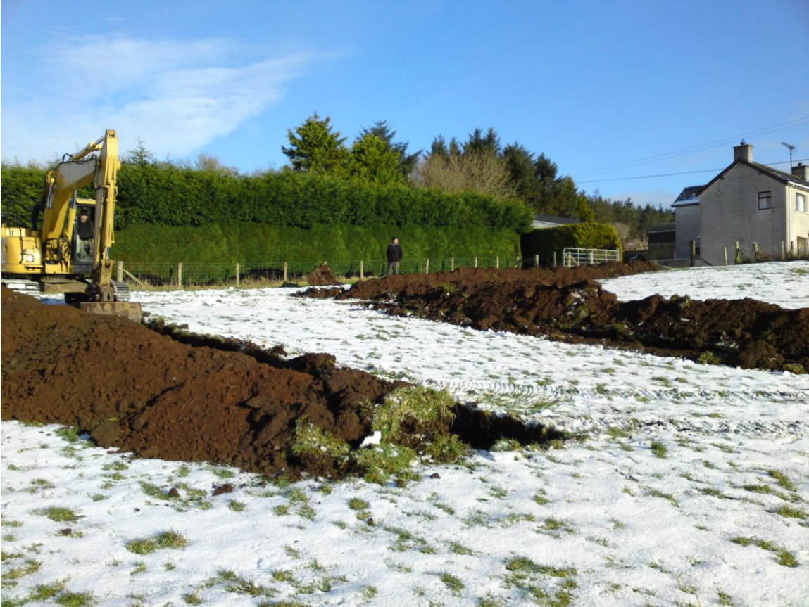
Plate 5: View of the application site following the excavation of the three evaluative test trenches, looking north-east.
